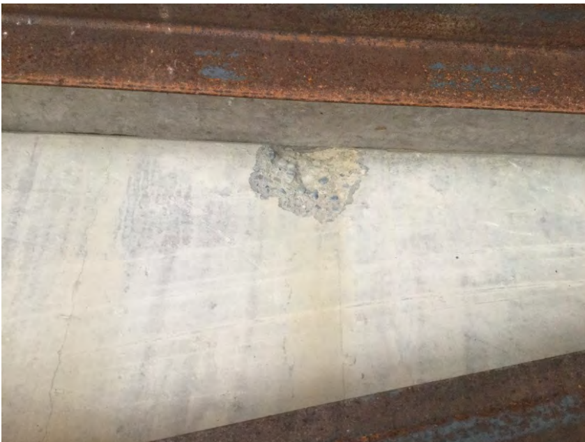
Small spall at left bank ballast wall
